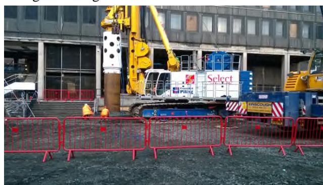
Figure 3 - Bauer BG42 Piling Machine with Segmental Casing Installing Test Pile and Anchors
