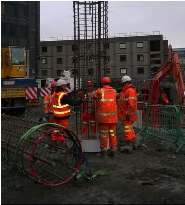
Figure 5 below shows the 14MN pile testing frame that was used to test the pile.
